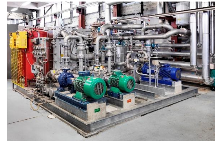
HIPA cooling circuit with recovery
